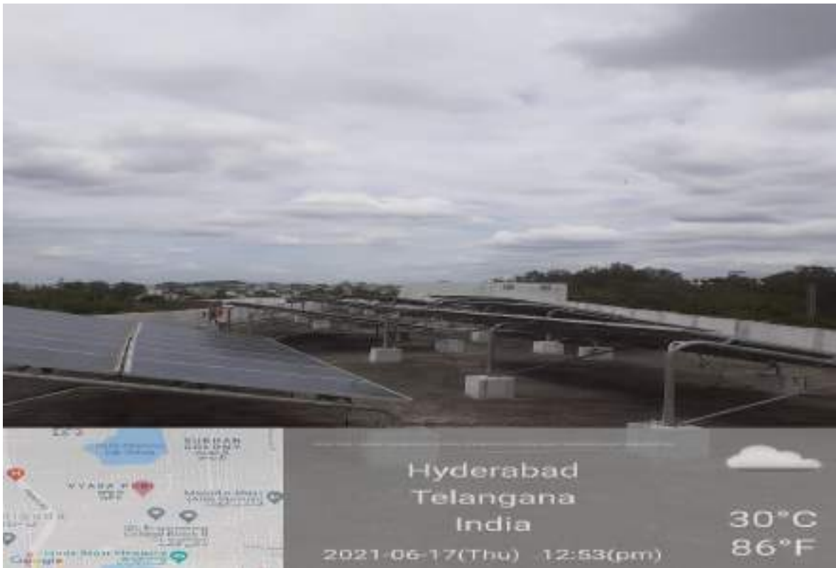
A view of MIST 100kW solar power plant
